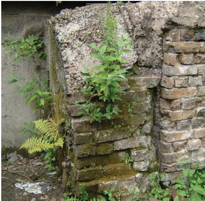
Figure 27 probable remains of the Hewett's Icehouse walls at base of Wigzells building (source: the writer)
